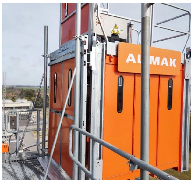
Genelba Thermoelectric Power Plant, Buenos Aires, Argentina
