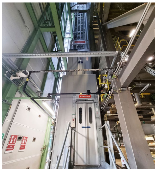
SSE Great Island Power Station, Ireland
