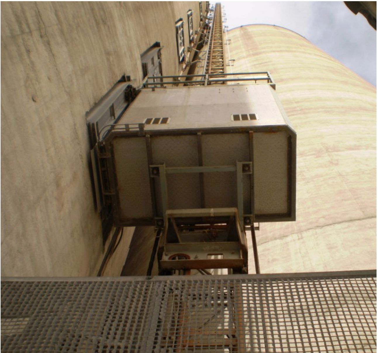
Graincorp Grain Handling Facility, QLD, Australia
