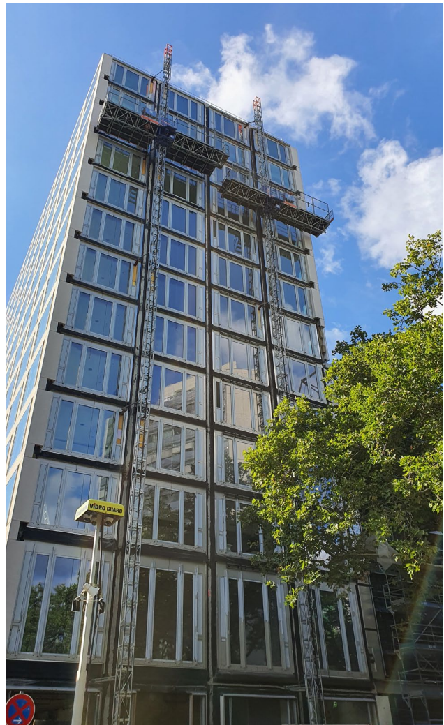
Ten Alimak mast climbing work platforms at work on the facade of the DGB tower in Berlin, Germany
