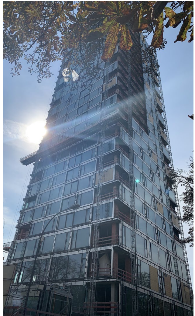
One of the eight Alimak MC 450 mast climbing work platforms at work on the 160 Park View construction project in Frankfurt am Main, Germany
