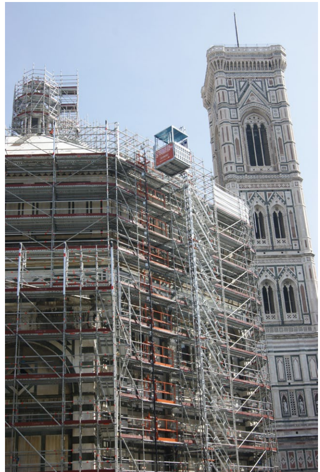
Alimak TPL enhanced productivity during the restoration of the art treasure Baptistery of San Giovanni.
