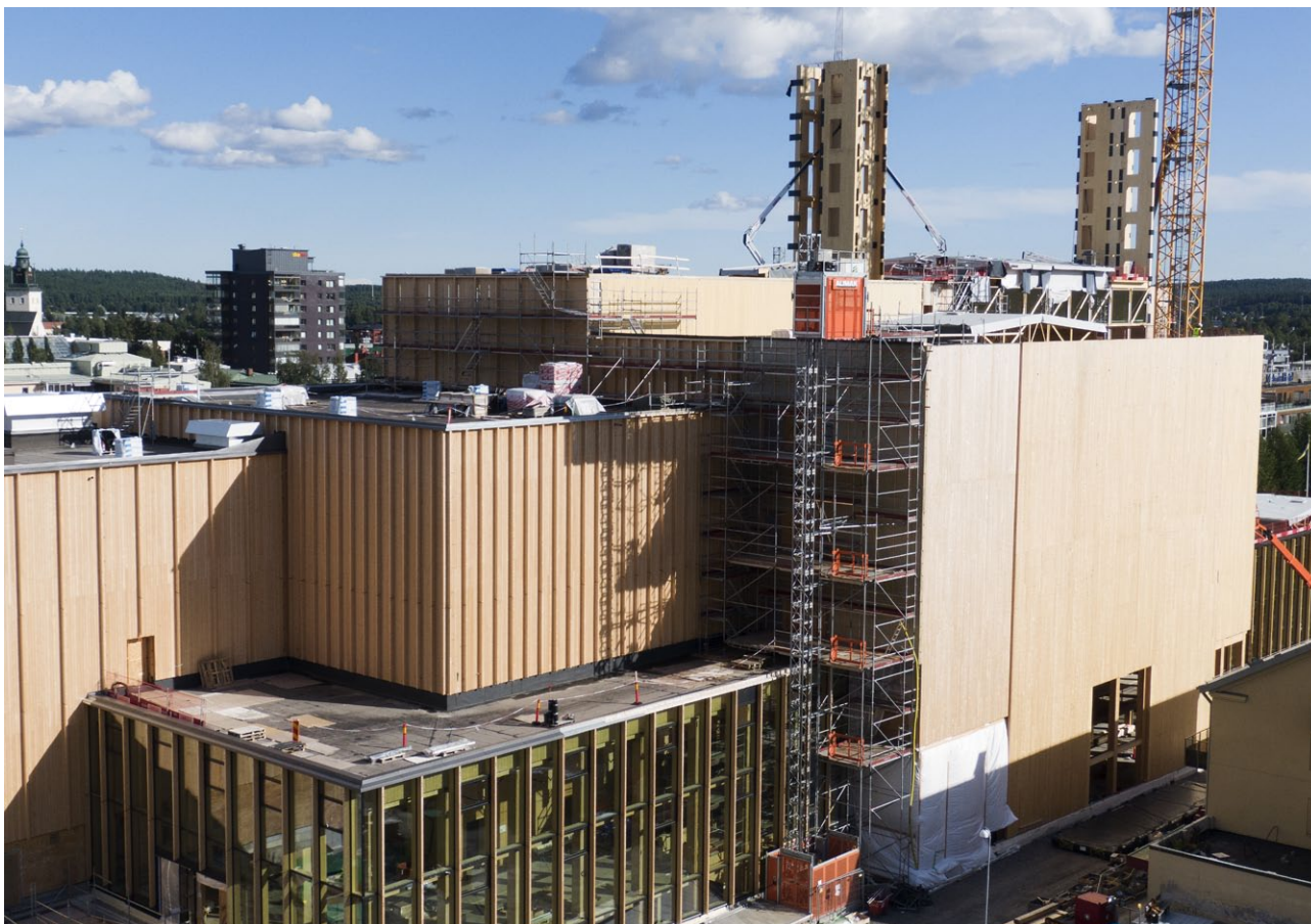
Alimak hoists and work platforms at the construction of The Sara Cultural Centre in Skellefteå.
