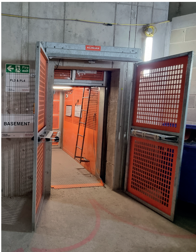
One of the Scando 450 FC hoists, installed in a lift shaft.
